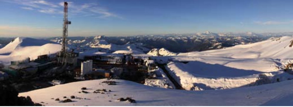
Estrella pad and sump. Courtesy of Estrella.
