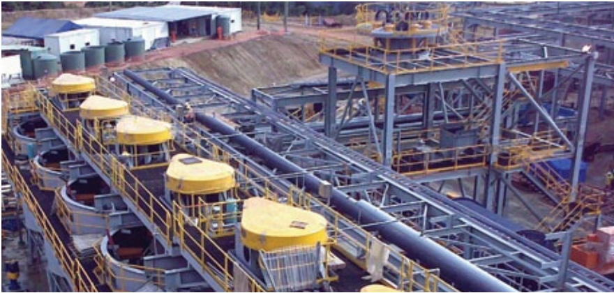
Flotation tanks at Hidden Valley mine, Morobe province. Photo courtesy of Kramer Ausenco.
