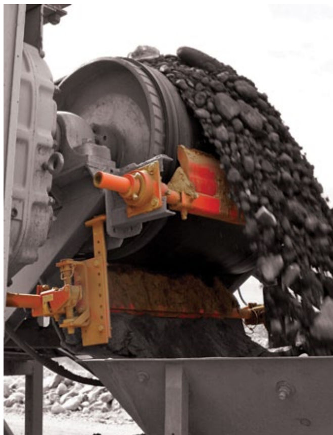
Belt cleaners. Photo courtesy of Martin Engineering.
