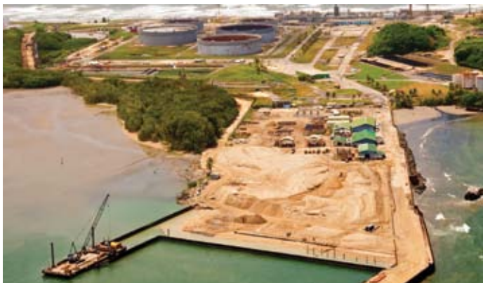
Port at Galeota under construction. Courtesy of National Energy Corporation of Trinidad and Tobago Limited.
