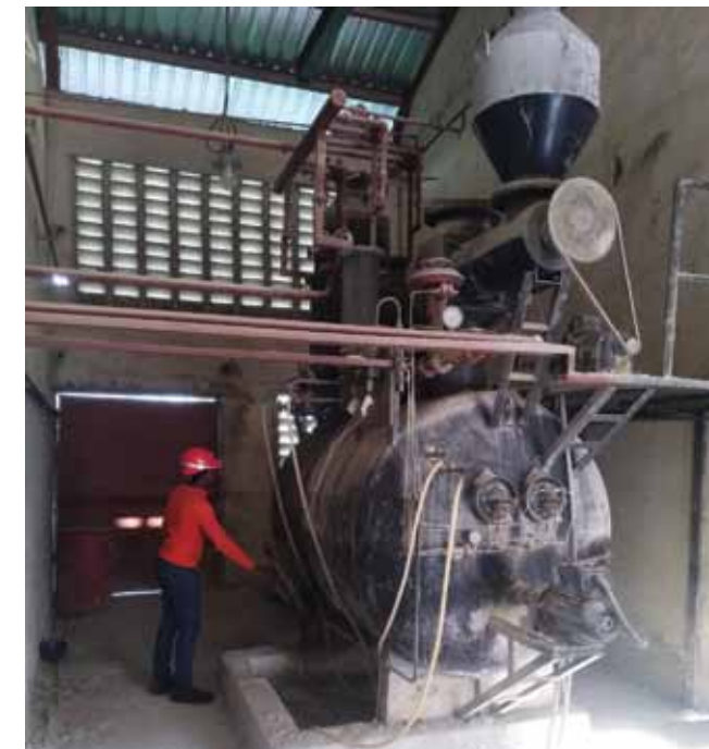
Acetylene gas plant, photo courtesy of Hopeup Integrated Industries.
