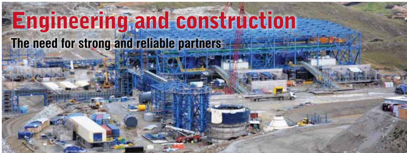
The completion of Constancia, Las Bambas and Cerro Verde may open a period lacking new large construction projects in Peru's mining industry. Photo: Las Bambas concentrating plant under construction, courtesy of MMG.
