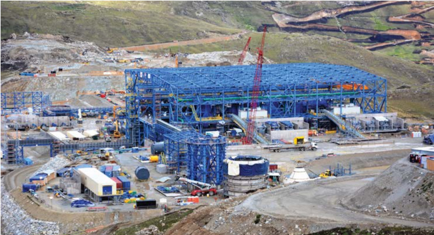
Peru's copper production will continue its upward trend moving forwards. Photo: Las Bambas concentrator plant under construction, courtesy of MMG.
