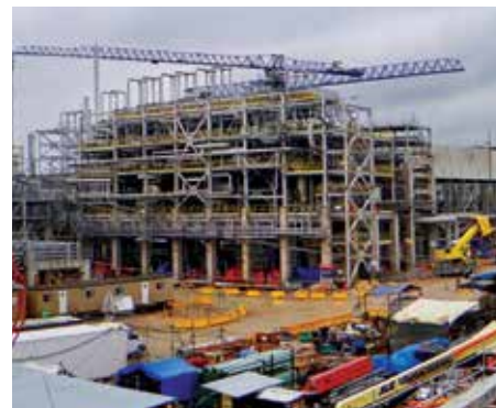
Hot water handling unit and compression unit of LDPE plant. Photo courtesy of Maire Tecnimont Group.
