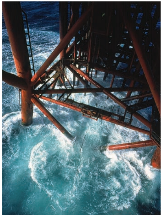
Winds of 50 miles per hour or more in the North Sea make for sea action on platform risers. (Photo by Lowell Georgia.)
