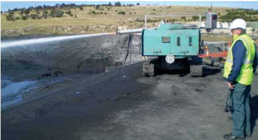
Cannon and operating staff for Superior Coal, specialized in coal waste management solutions. The vast majority of their projects have been located in the rich coal belts of the Hunter Valley in New South Wales and Bowen Basin in Queensland. (photo courtesy of Superior Coal Limited)
