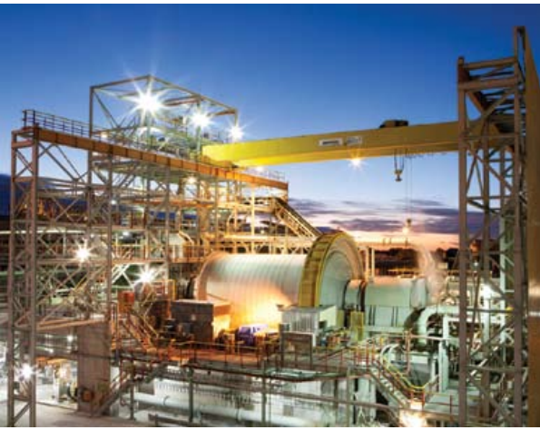
Moab Khotsoeng metallurgy plant South Africa. (Photo by Annalien Swanepoel, courtesy of AngloGold Ashanti)
