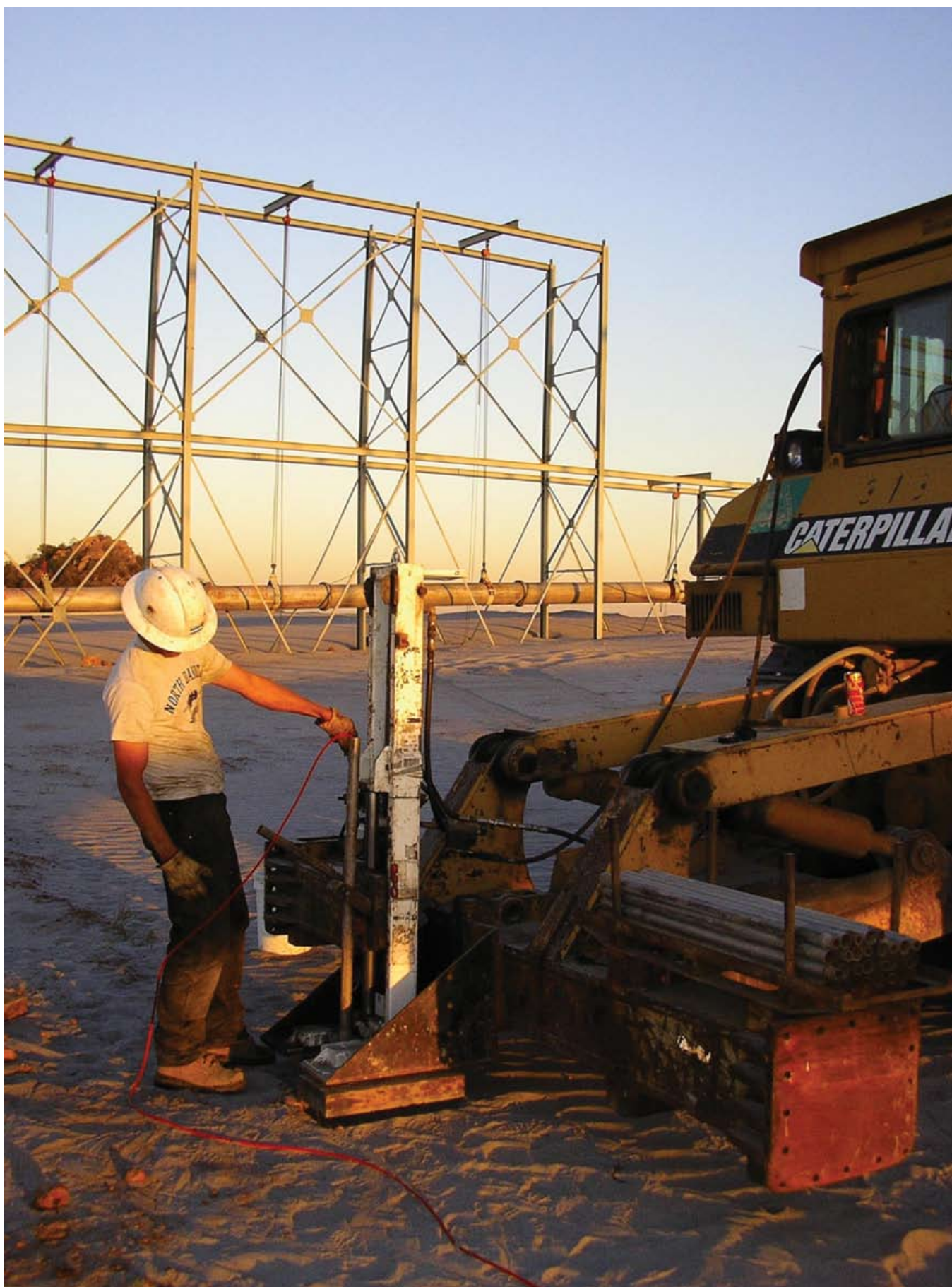
Piezococone (CPT) Probing at Palaborwa Mining Company (Photo courtesy of Knight Piésold)
