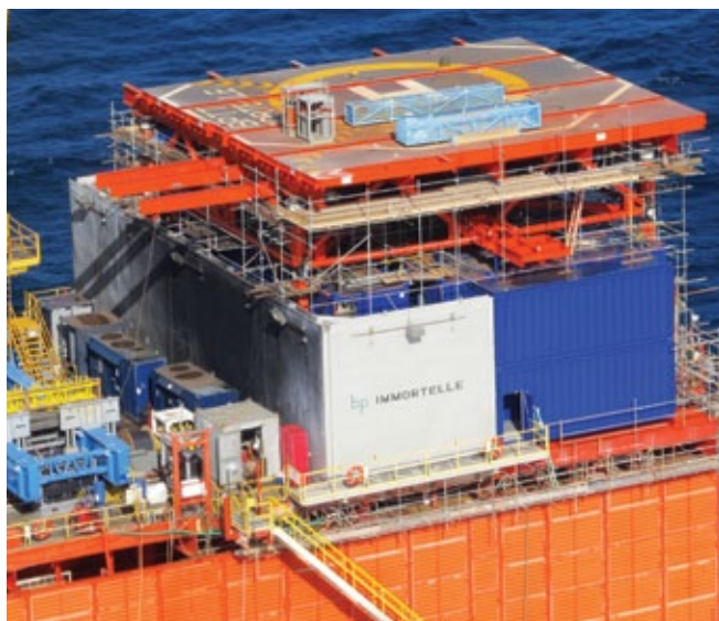
BpTT's Immortelle Quality of Life Helideck Fabrication at Carillion's yard in Waterloo.
