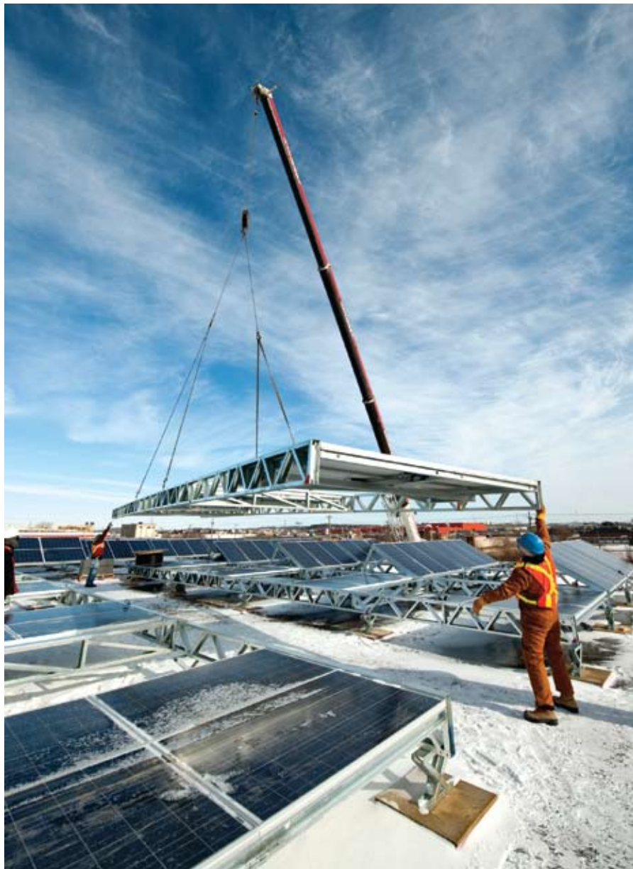
3. Winter sun. Canada’s first 250-kW rooftop solar installation, in Cambridge, Ontario. Courtesy: AECOM
