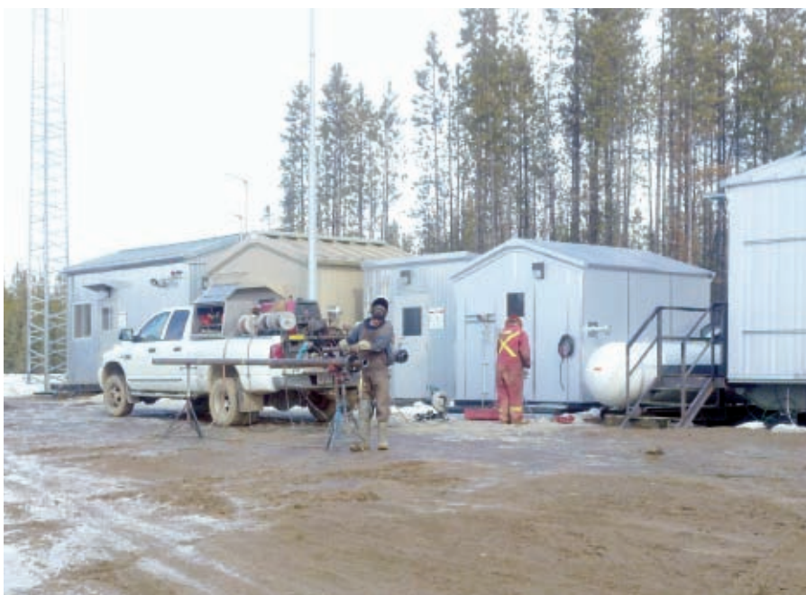
Generators and office buildings at Dejour Energy's Woodrush operations in the Peace River Arch, British Columbia.
