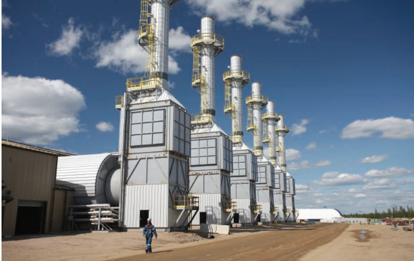
Steam boilers at Cenovus Energy's Foster Creek operations in northeast Alberta.
