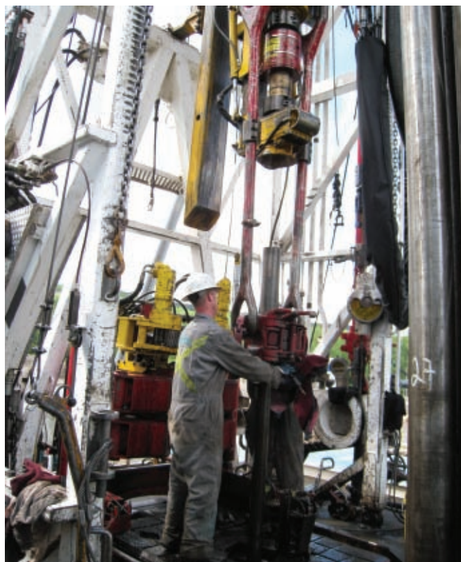
Trinidad Drilling's Rig #46 operating in the Montney shale in northeastern British Columbia.
