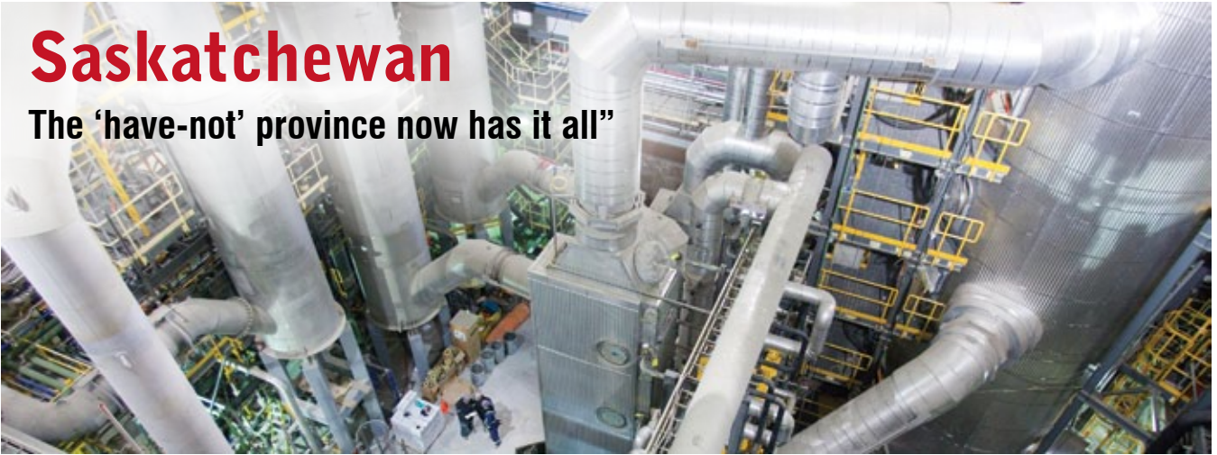
Aerial view of some of the piping Graham fabricated and installed at Cameco's Key Lake acid plant. Photo courtesy of Graham.
