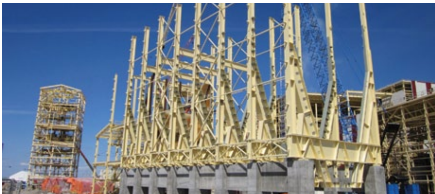
PCS Rocanville West Expansion, Rocanville, SK - Rocanville includes over 20,000 tons of steel, including fabrication and erection of support buildings and loadout. Photo courtesy of Supreme Steel.
