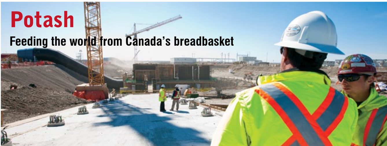
Mosaic project manager Steve Grinius surveys the K3 site with an employee from PCL. Photo courtesy of The Mosaic Co.
