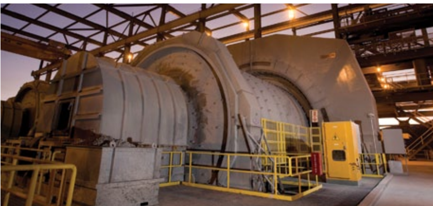
Ball mill located in the Cerro Verde concentrator plant. Photo courtesy of Cerro Verde.
