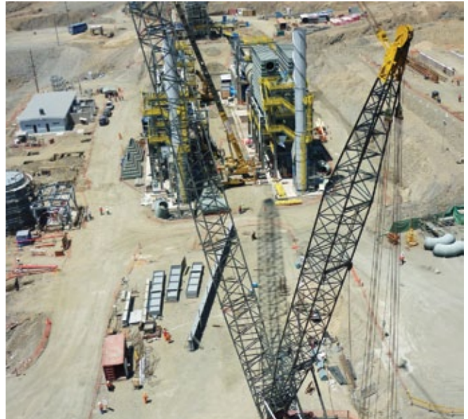
Engineering and construction firms fight for Peru's juicy contracts. Photo courtesy of Stiglich.
