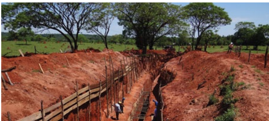
New Trend trench located on the Discovery Trend at the Paso Yobai project, Paraguay. (Photo courtesy of Latin American Minerals).
