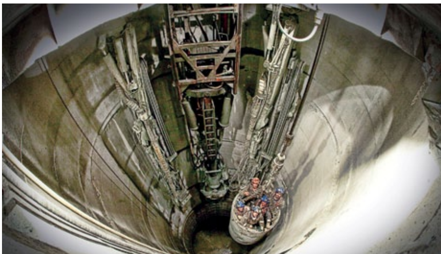
Dumas crew being transported during shaft sinking. (Photo courtesy of Dumas Mining).
