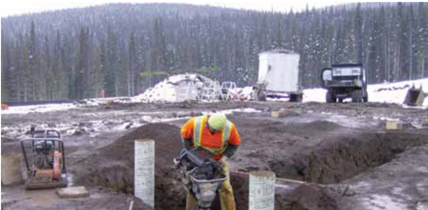
Construction of the foundation for the water treatment plant at Metal Mountain Resources' Dome Mountain mine.
