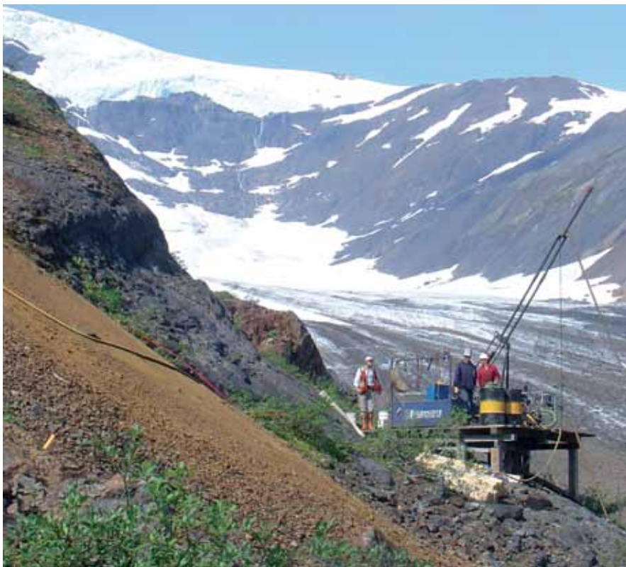
Drilling at Bravo Gold Corp.'s 100%-owned gold and silver Homestake Ridge project near Stewart BC. (Photo courtesy of Manex Resources)
