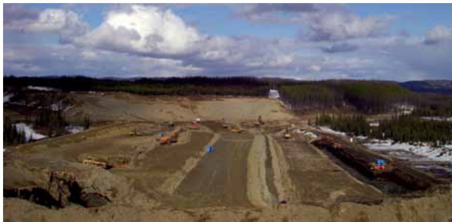
Knight Piésold designed the mine waste and water management plan and is providing QA/QC support during the construction for Mt. Milligan.
