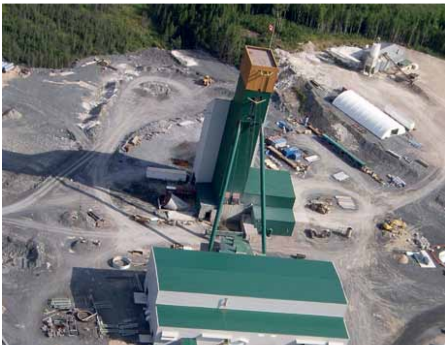
Merit Consultants were the construction managers of Red Lake mine and subsequent McEwen shaft expansion projects, Ontario (Goldcorp Inc.)
