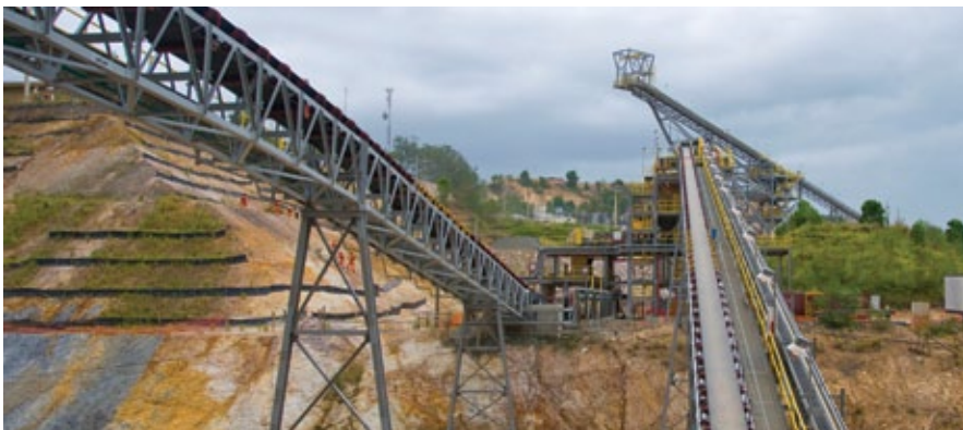
Pueblo Viejo Gold Project in the Dominican Republic (Owner: Barrick Gold Corporation). Photo courtesy of Fluor.
