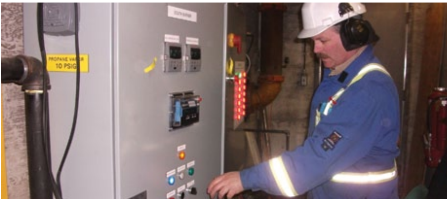
Superior Propane technician making up set-up adjustments to a vaporizer and pump system. Photo courtesy of Superior Propane.
