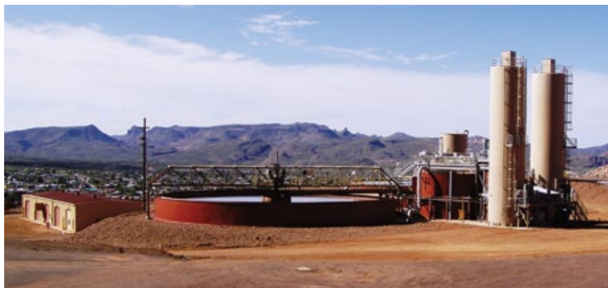
Resolution copper HDS plant. Photo courtesy of CH2M HILL.
