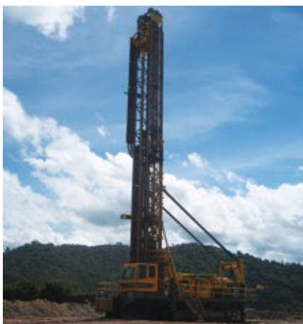
Atlas Copco drill rig operating on a site in the northern region of Brazil. Photo courtesy of SRK.
