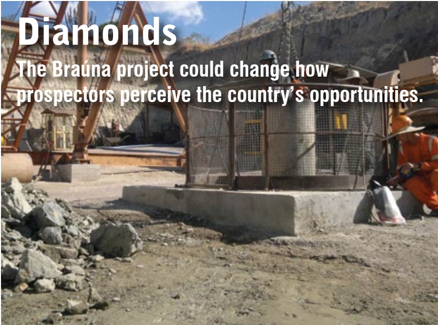
Samples of kimberlite being mined from Lipari's 100 m deep bulk sample shaft excavated into the BR3 kimberlite pipe. Photo courtesy of Lipari.
