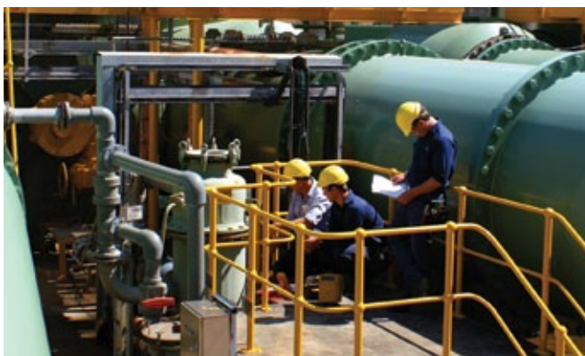
Condenser Cooling Water Piping. Photo courtesy of Eraring Energy.
