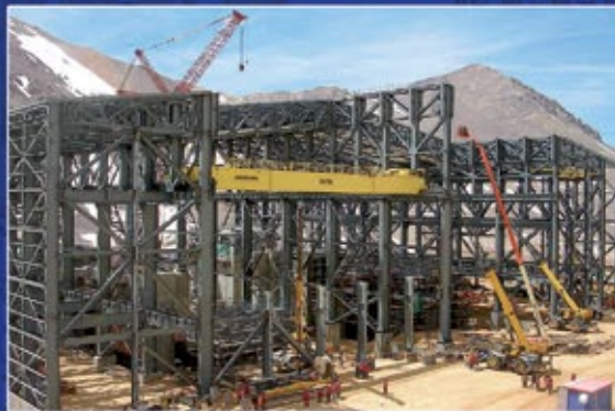
Pascualama grinding building, 7,300 Tons, Barrick
