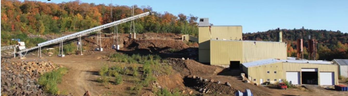
Kearney mine's ore stacking conveyor and processing plant. Photo courtesy of Ontario Graphite.
