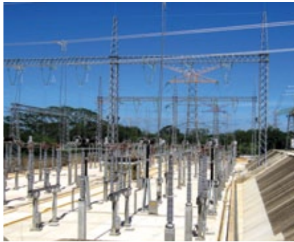
400 kV Substation Julie - Veracruz | Mexico, Courtesy of Isolux
