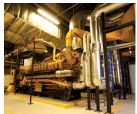
The CHP system powered Cat can provide 11.2 MW of electrical energy
