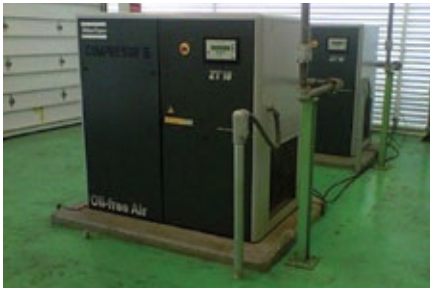
Manufacturing Excellence: Air Compressor in the Mexico City factory of Atlas Copco
