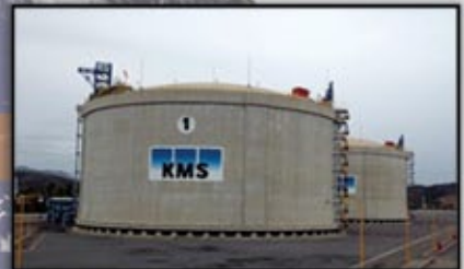
Mitsui developed a LNG regasification terminal in Mexico, and is a part of its sponsor group.
