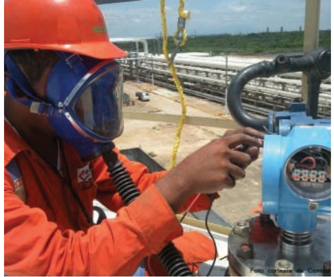
A worker installs transmitters on equipment in Mexico. (Courtesy Controflux)
