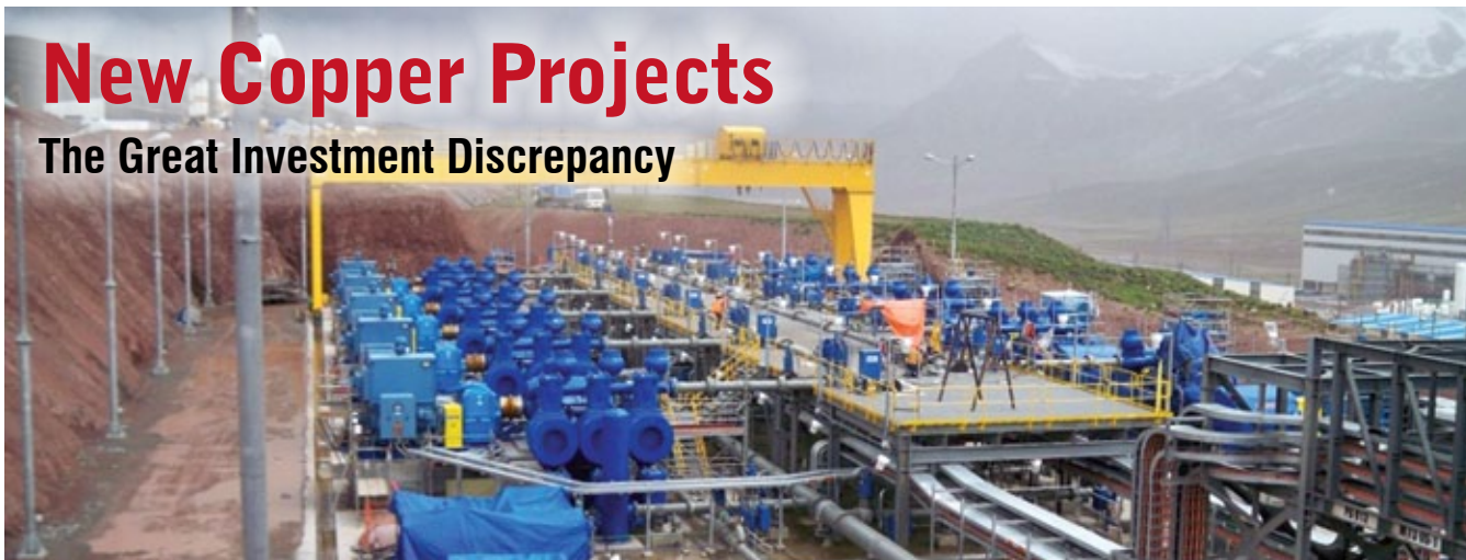
Brass completed the basic and detailed engineering for the tailings pump station and distribution pipeline. Presently, the system is in pre-operational phases: mechanical completion, pre-commissioning, commissioning, and start-up. Photo courtesy of Brass.
