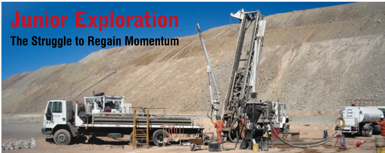
After rising steadily for the best part of a decade, exploration activity in the country dropped by some 60% between 2012 and 2013. Photo courtesy of Codelco.
